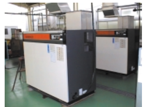
Newly installed compressors (one with an inverter and one with an automatic start/stop function, both having a capacity of 37 kW)
